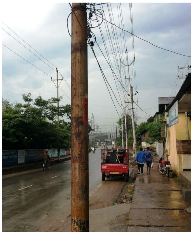
33 kV line inside city area of Assam
