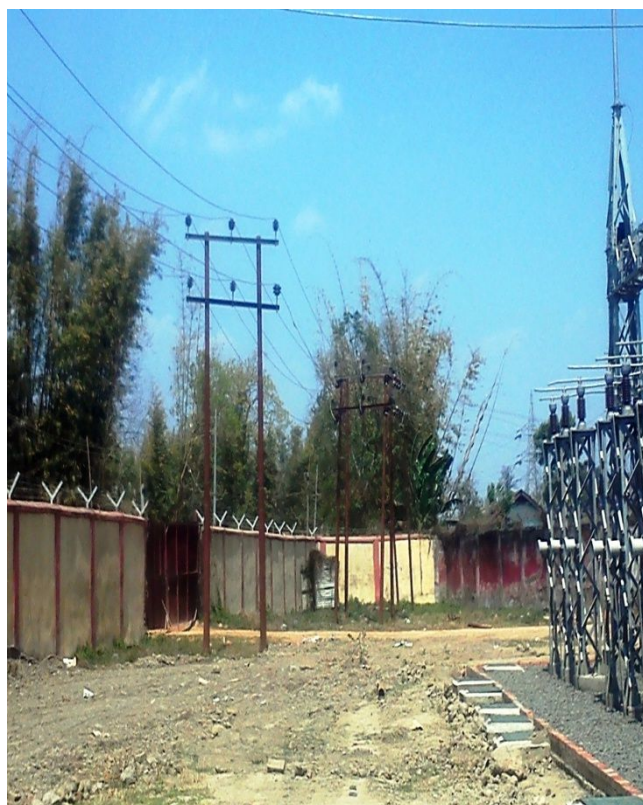
33 kV (H Pole) line inside substation
